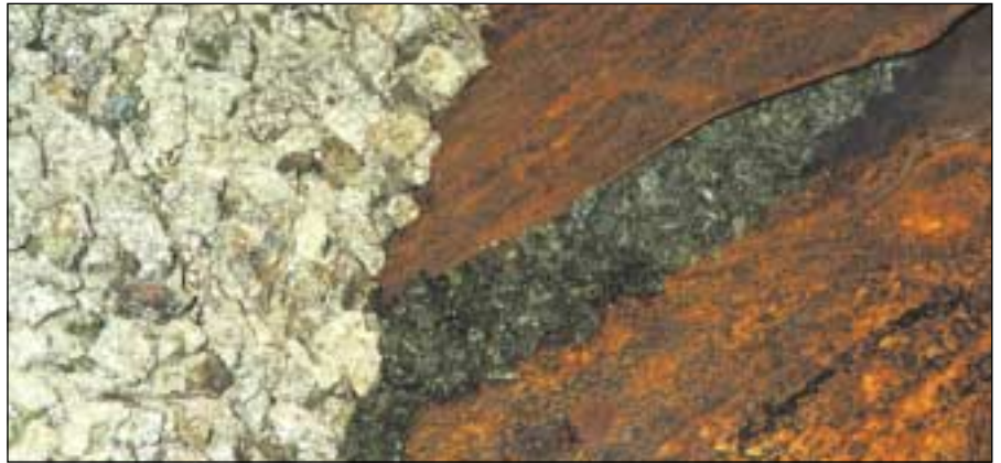
Steel partition failures can have far-reaching consequences
