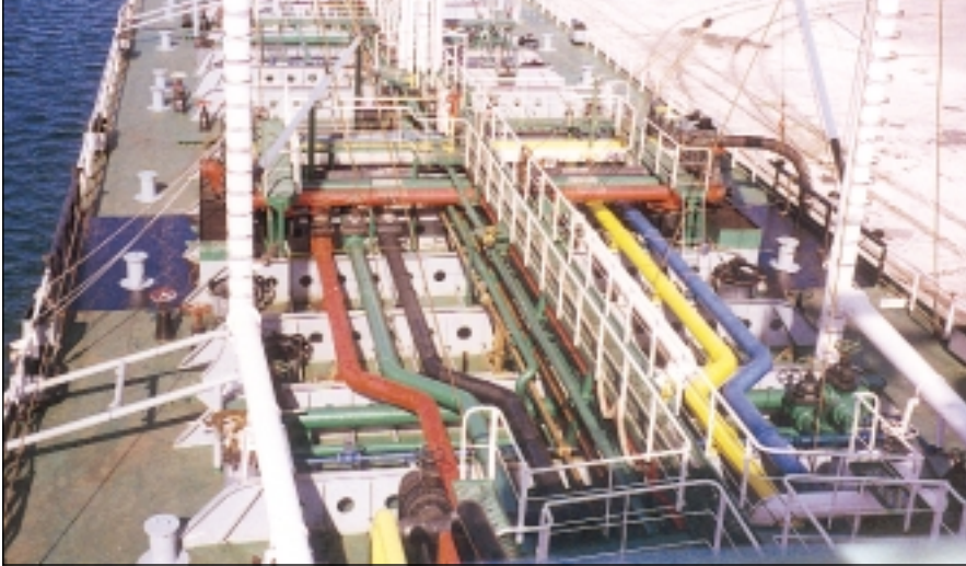
Ships' officers should have a good knowledge of their vapour line systems
