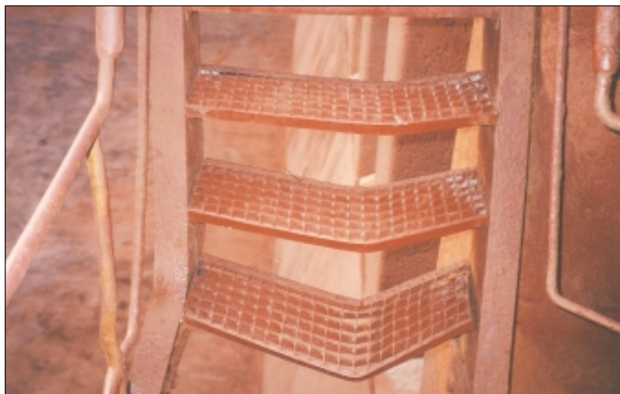
The structural condition of ladders is one of a number of recurring deficiencies in incidents reported to the Club.
