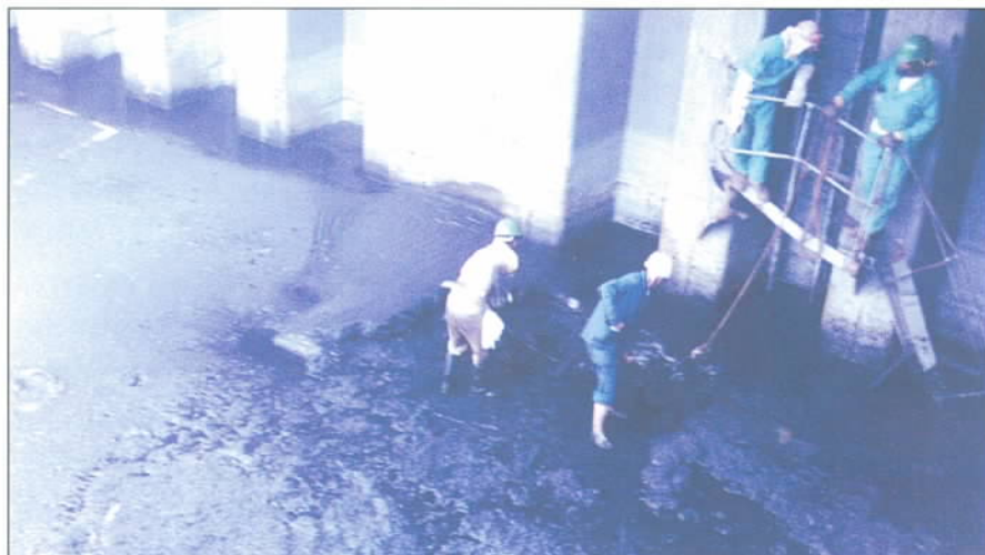
The consequences of failure to conduct regular soundings can be far-reaching
