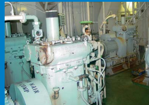
▶ Typical air compressors on a vessel
